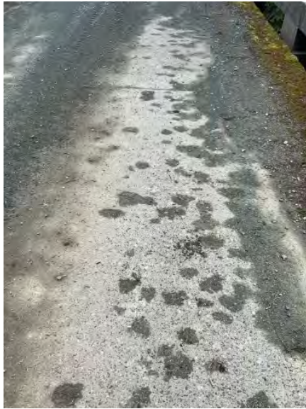
Growser damage to deck surface
